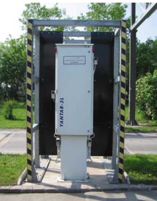
Installed radiation monitors automatically detect the presence of radioactive material. © Stefan Schönhacker, WIRK.ZONE www.wirkzone.at
